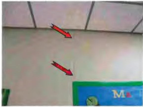
Photo #46 Crack in gypsum wallboard wall
