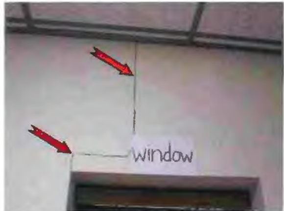
Photo #58 Crack in gypsum wallboard wall
