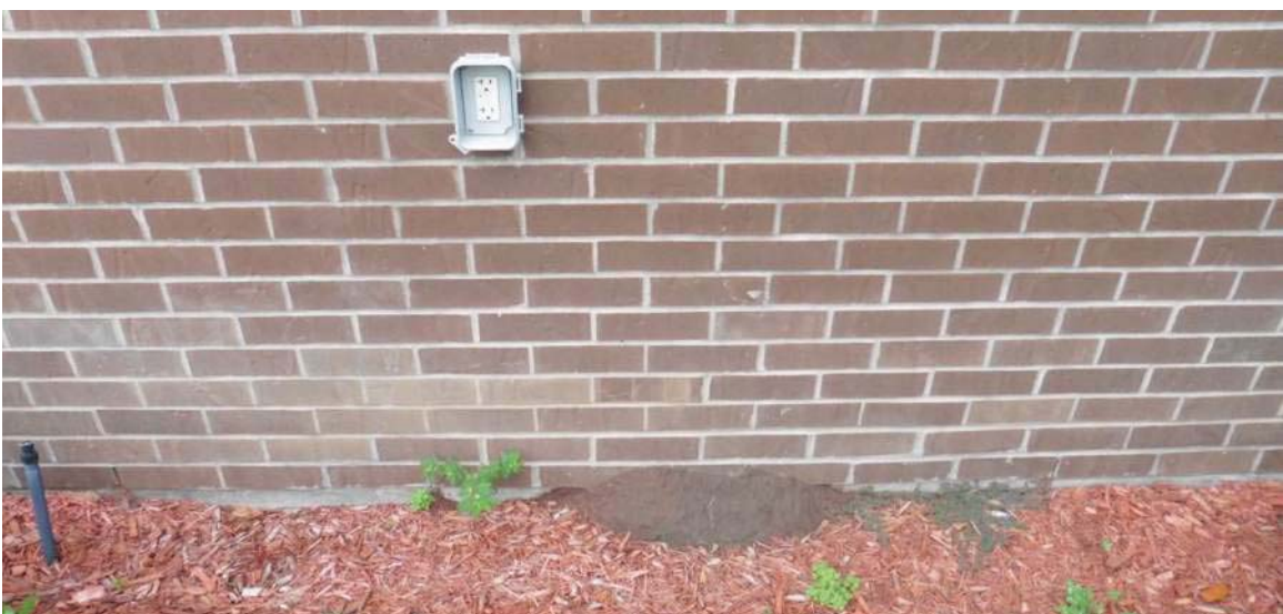
Insect infestation, and example of unprotected electrical
