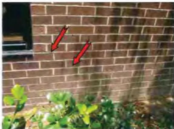
Photo #19 Masonry-mortar-joint crack
