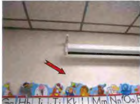
Photo #68 Crack in gypsum wallboard wall
