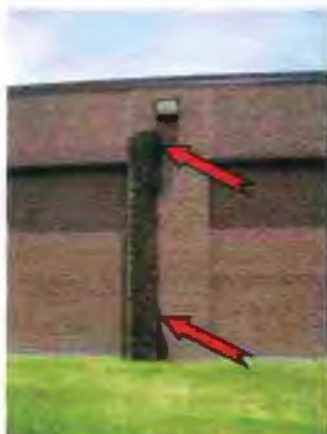
Photo #23 Staining on exterior brick veneer
