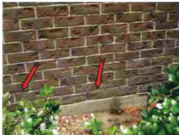
Photo #22 Masonry-mortar-joint crack
