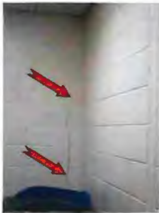
Photo #25 Crack through concrete masonry unit wall
