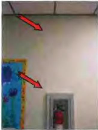
Photo #43 Crack in gypsum wallboard wall
