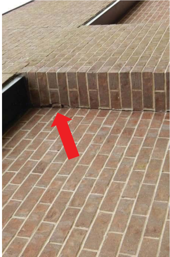
#11 Cracked brick at end of inset panel.
