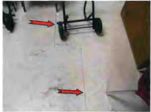
Photo #50 Separations in vinyl tile floor
