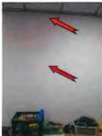
Photo #59 Crack in gypsum wallboard wall
