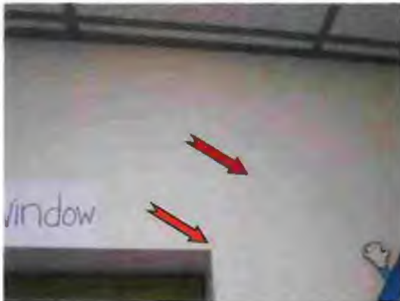
Photo #57 Crack in gypsum wallboard wall
