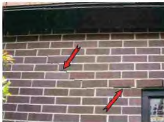
Photo #20 Masonry-mortar-joint crack
