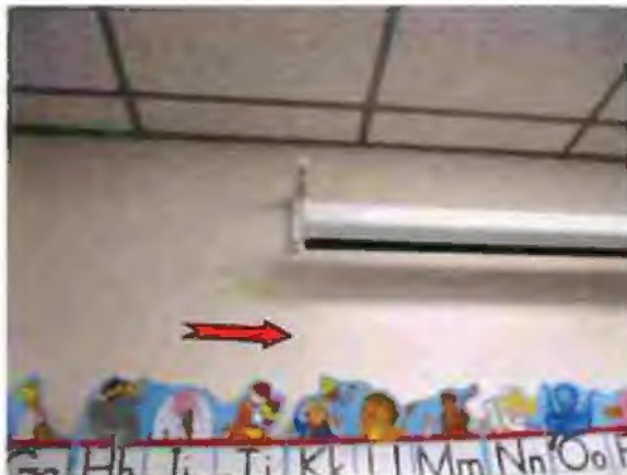
Photo #55 Crack in gypsum wallboard wall
