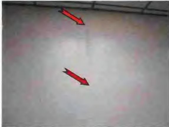
Photo #67 Crack in gypsum wallboard wall
