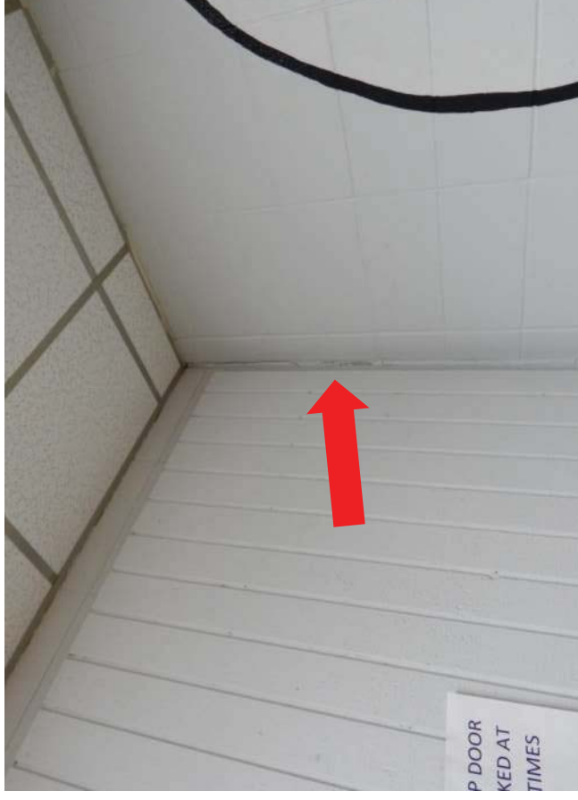
#47 Crack in corner of CMU wall
