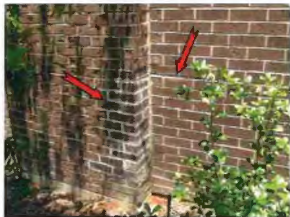
Photo #21 Masonry-mortar-joint crack
