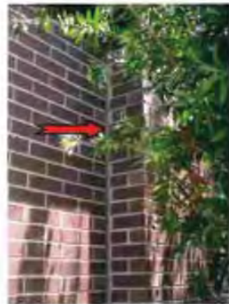
Photo #18 Separation at expansion joint
